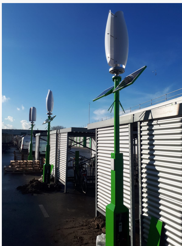
Wind and Solar E-bike Charging Poles
