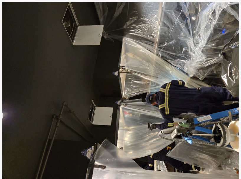
A Done Right hood cleaning specialist cleaning a commercial kitchen's grease filters and hood at a Japanese restaurant
