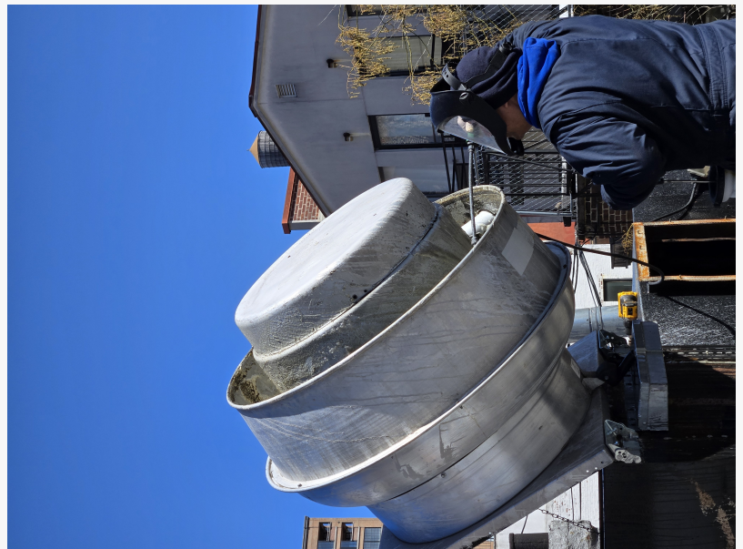
Grease doesn't stand a chance—expert hood cleaning high above Midtown keeps kitchens safe and city-compliant.
