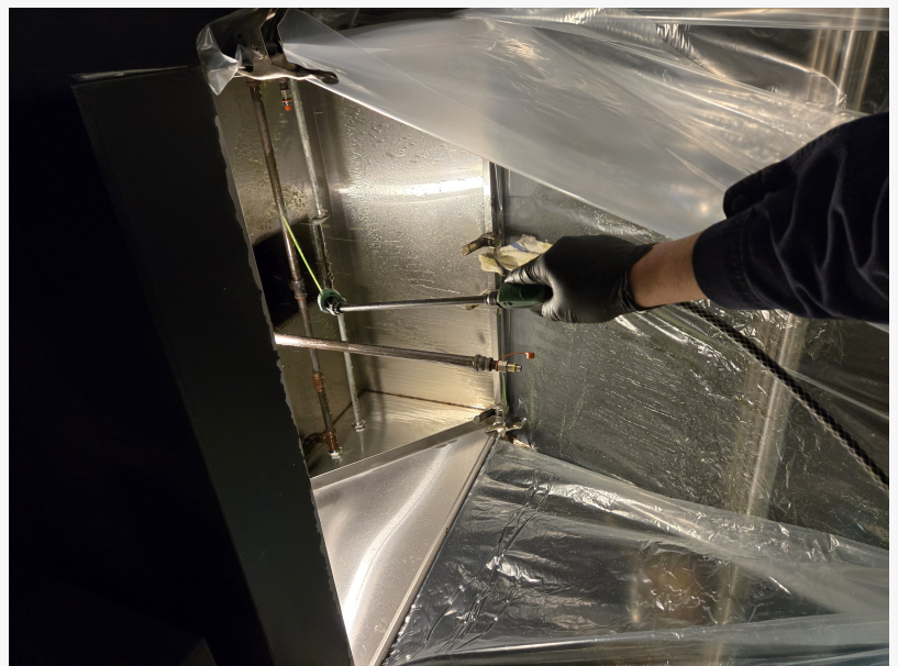
A Done Right hood cleaning specialist cleaning a commercial kitchen canopy at a local restaurant
