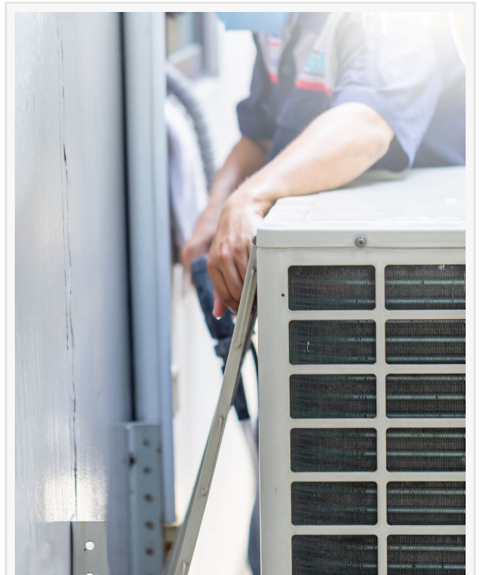
Filta Kleen Factory Licensed PCU Tech checking filters and prepping to repair them.
