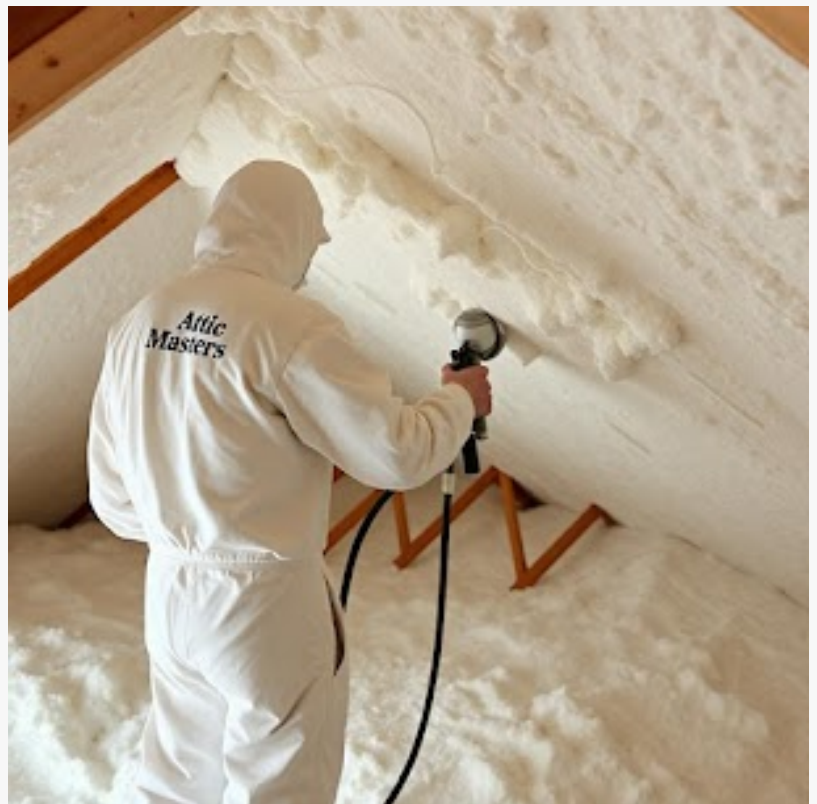
Attic Closed cell spray foam insulation
