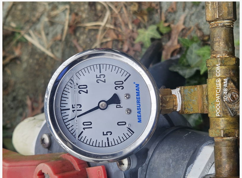
A Hidden Pool Pipe Leak Located
