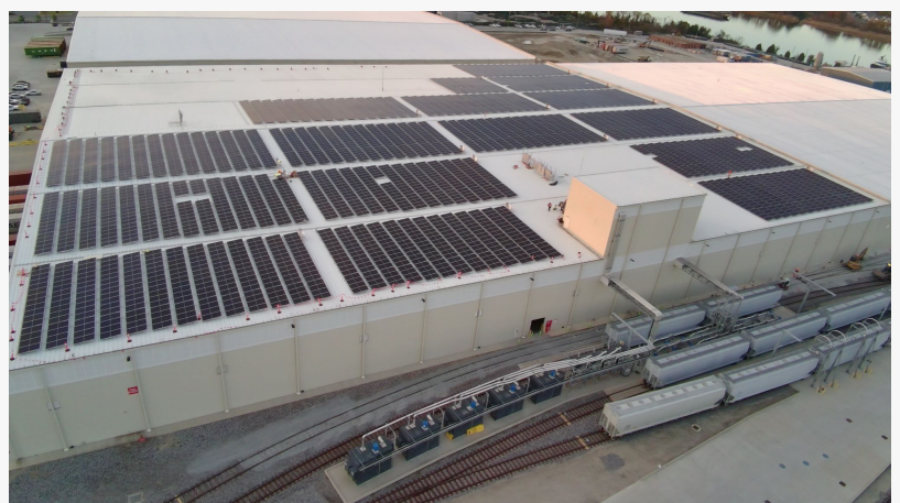
100MW Rooftop Commercial Solar Project
