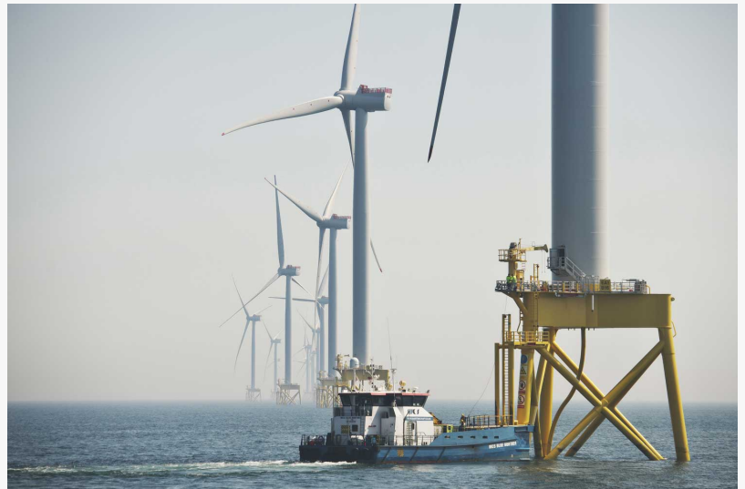
Scottish Power's East Anglia One wind farm
