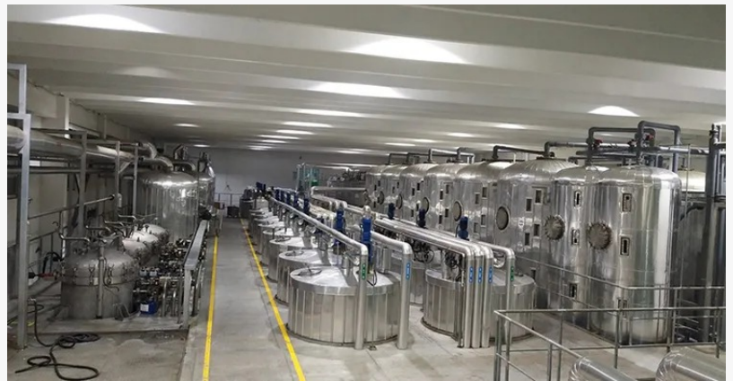
Sorbitol Production Plant
