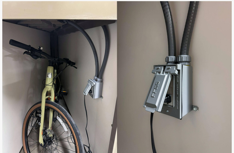
Today's modern ProPark locker with GFI outlet for e-bike charging.
