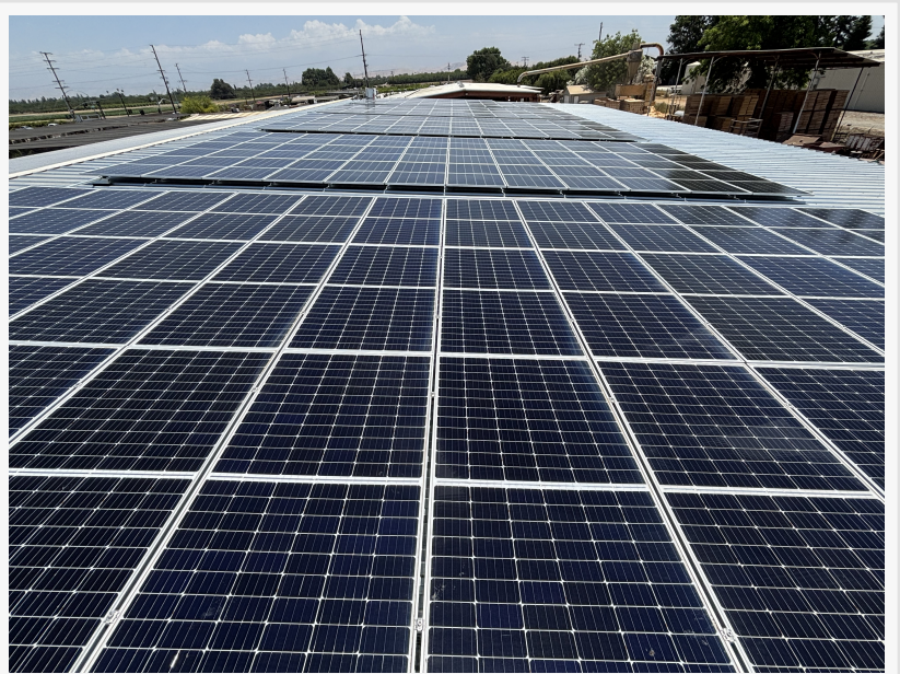
Solar Panel shining bright from a clean from Superior Solar Clean
