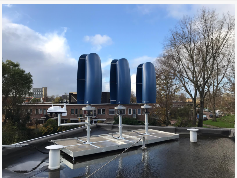
Three installed small size Wind Tulips
