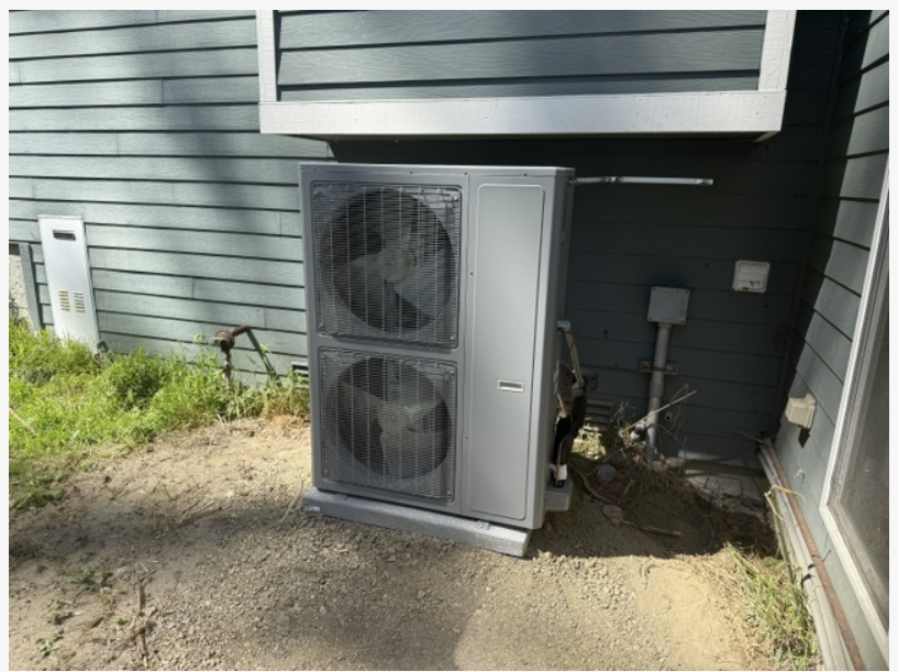
Heat pump newly installed by Mauro Electric Inc., showcasing the company's expanded full-service HVAC offerings.
