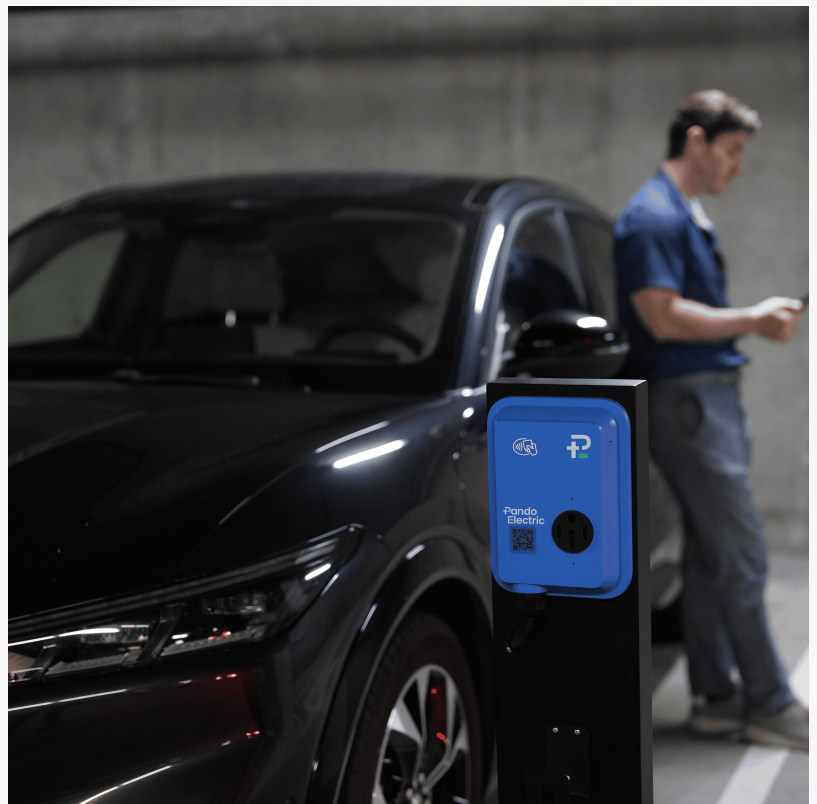
Charging up in a parking garage
