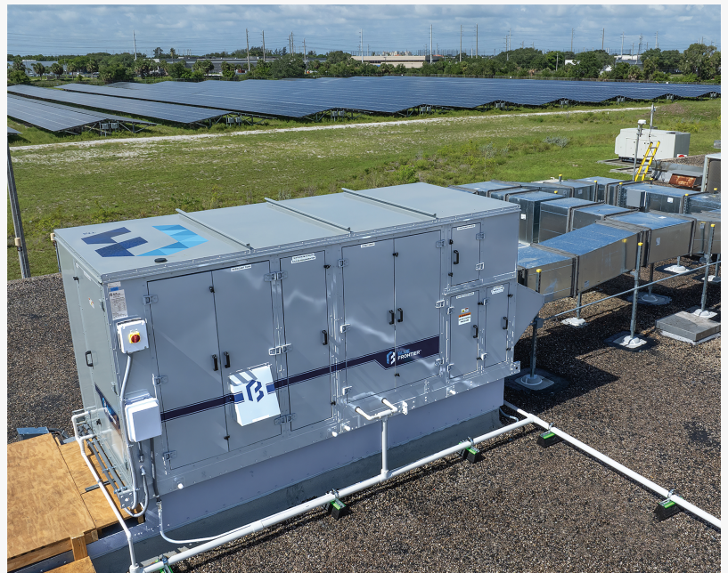
Blue Frontier's ultra-efficient AC unit storing solar energy and providing cooling for an office building in Riviera Beach, FL
