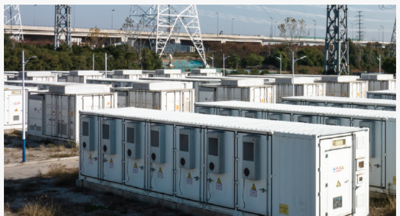
An energy storage system helping to power the grid.
