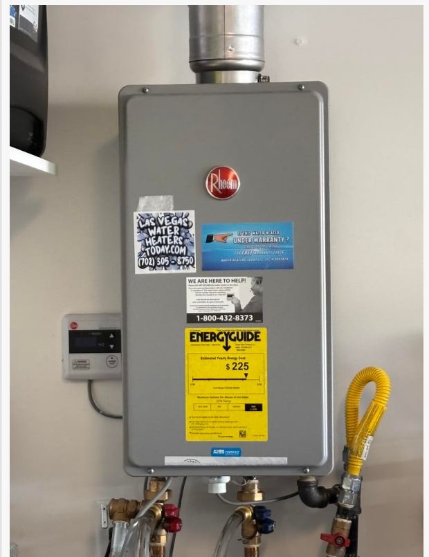
garage tankless water heater installation las vegas valley water heaters today
