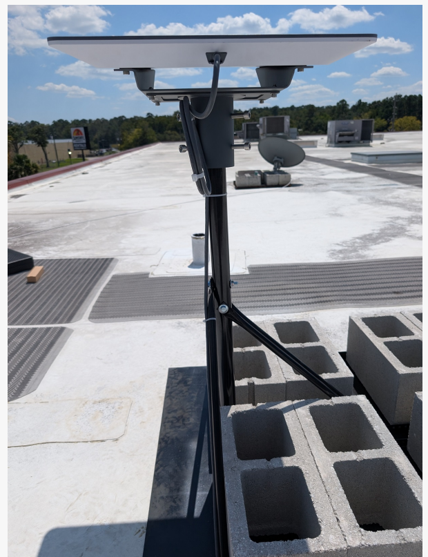
Starlink business installation Texas
