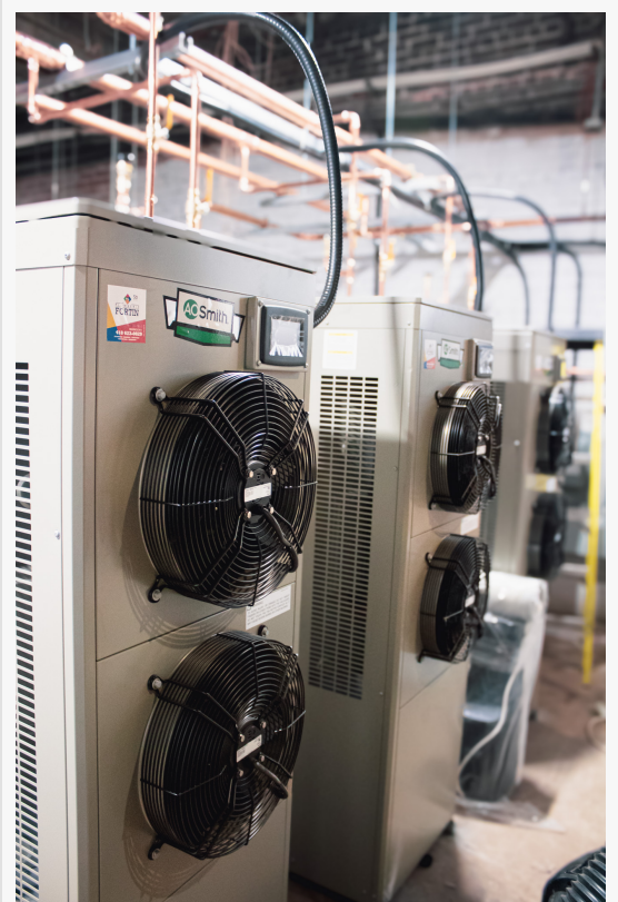
Energy efficiency in action: new high-performance equipment in the rental buildings of Société immobilière Bélanger in Québec and Lévis.
