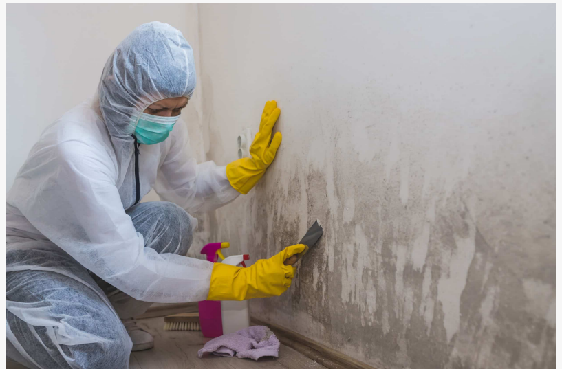
mold inspection in Annapolis
