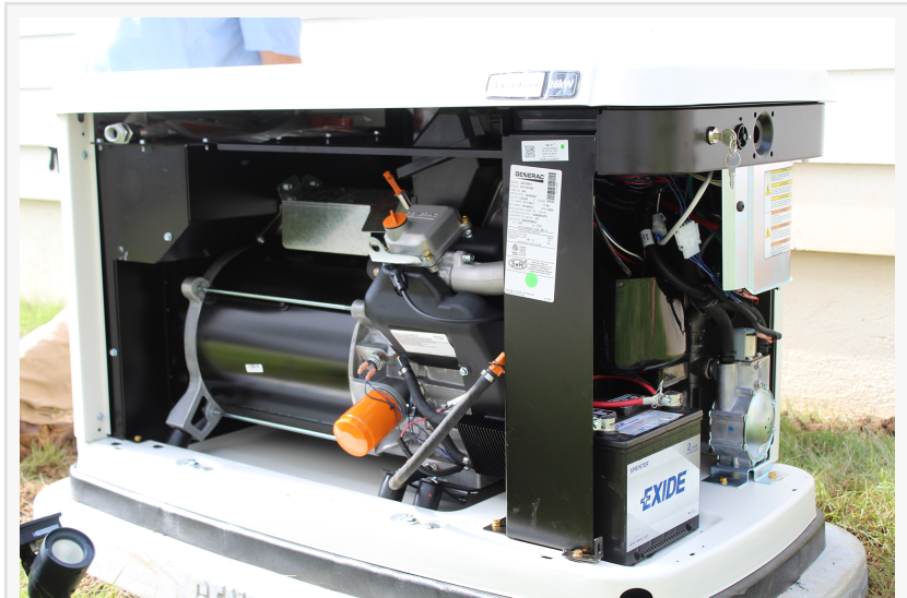
Home generator being serviced by Anderson Power Services
