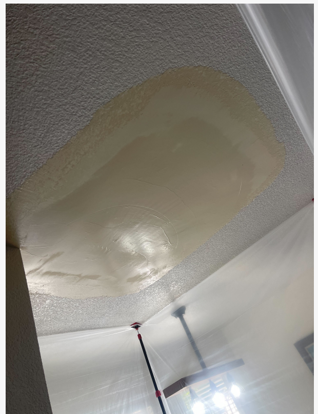
Water damaged patched and coated
