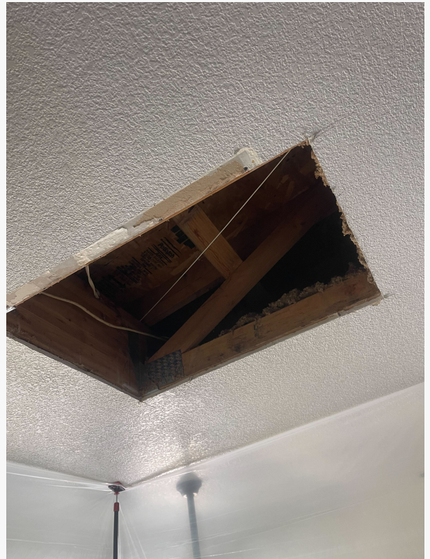
Ceiling water damage cut-out
