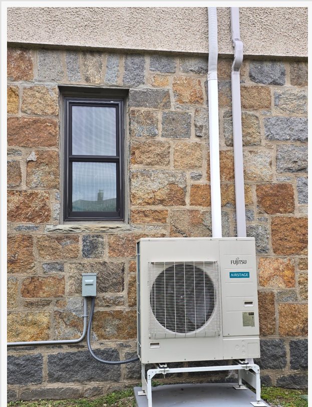
Whole Home Heat Pump installed in Milton, MA
