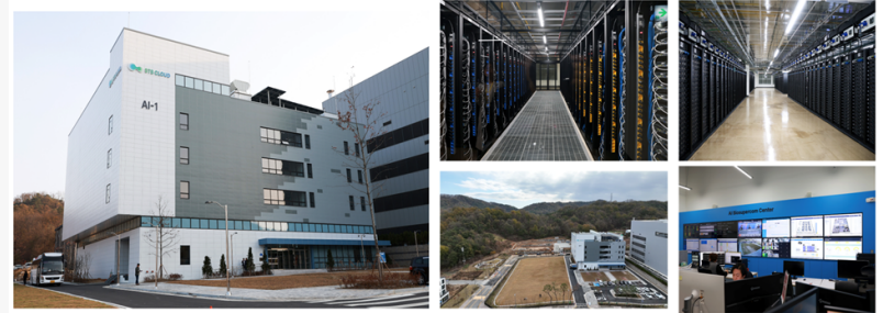
Syntekabio AI Bio Supercomputing (ABS) Data Center in Dungok, Daejeon
