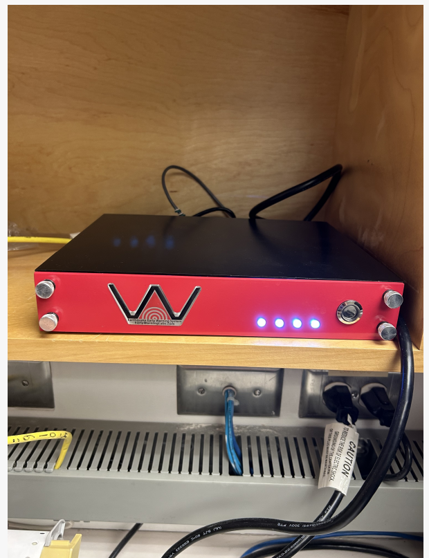
EWL Hardware on Site
