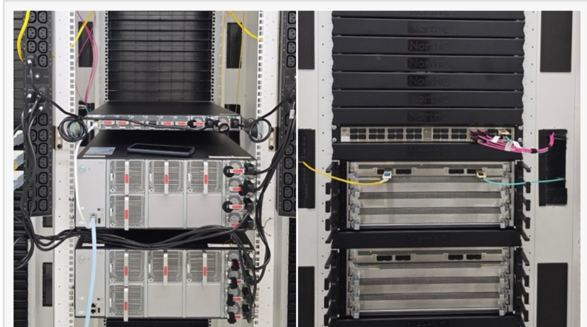
MIRhosting's 400G ZR+ network in Amsterdam — front and rear views of the active 4U network switches powering the upgraded colocation infrastructure.
