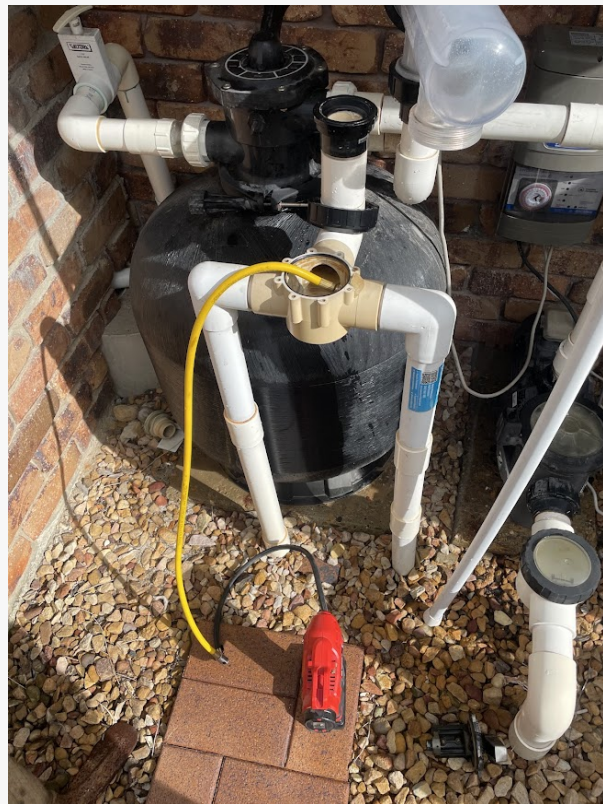
Pool Leak Detection method on pool for a client in Gold Coast by Leak N Pool
