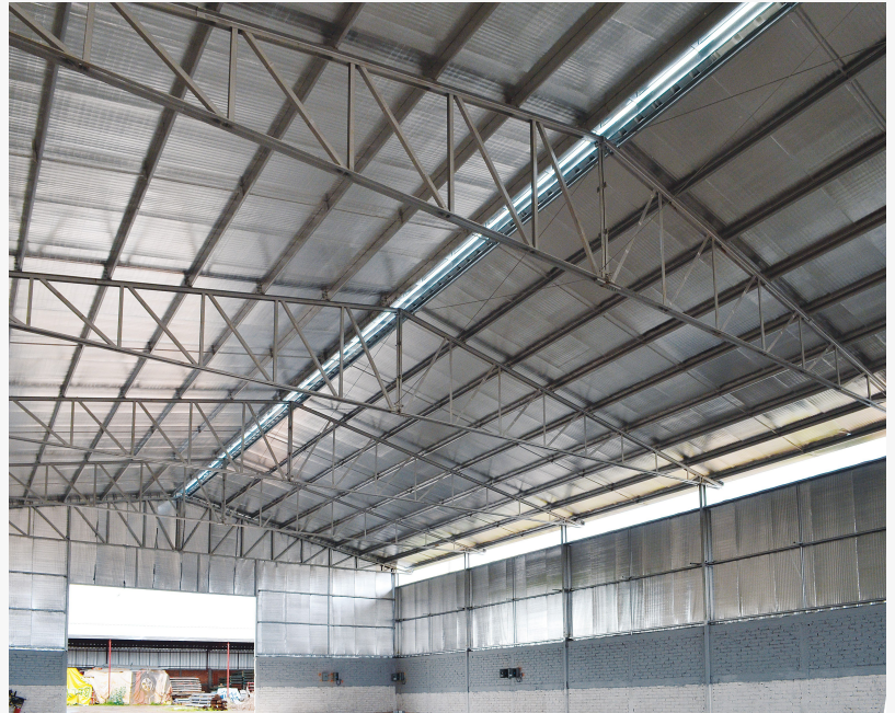
Prodex reflective insulation in agricultural building
