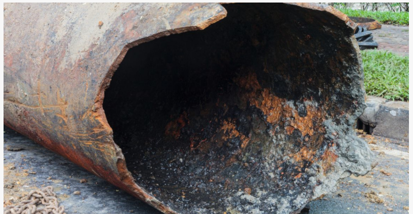
A close up look at cast iron pipe corrosion.
