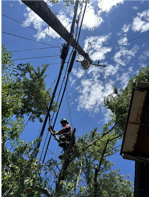
Tree Branches Falling Near Powerlines
