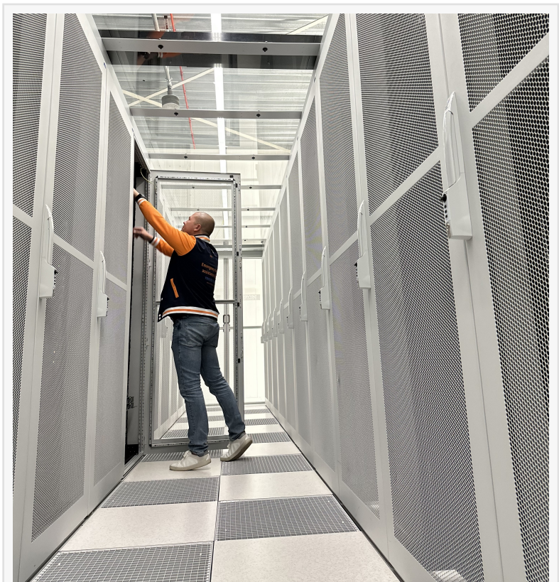
MIRhosting engineer at work inside the Amsterdam data center.
