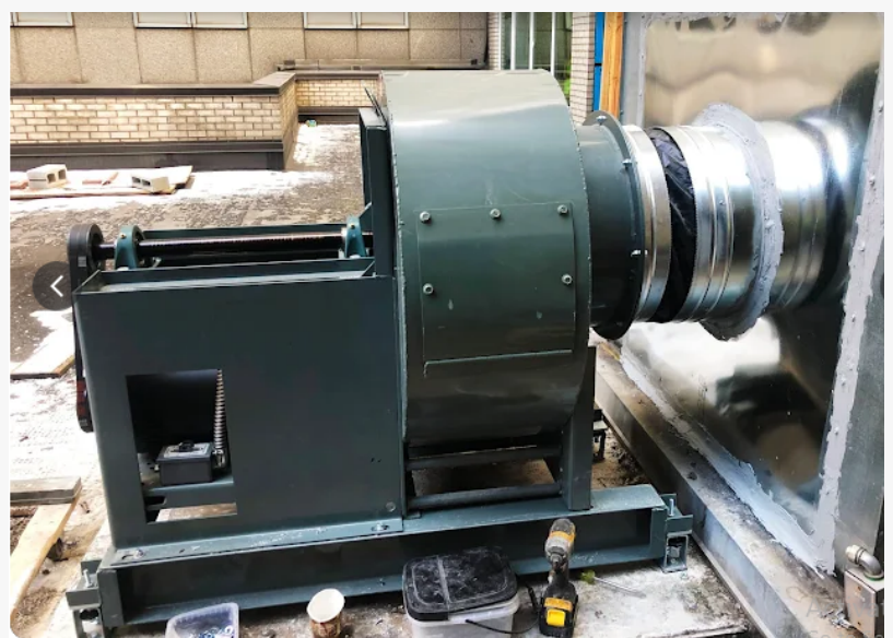
Rooftop Unit on Brooklyn building
