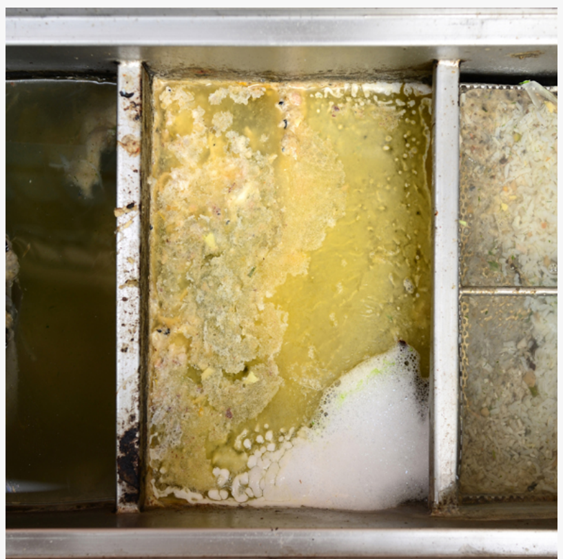
Fully loaded grease trap demonstrating the need for immediate cleaning to prevent FOG-related blockages.
