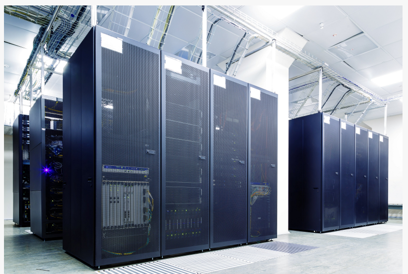
GPU & Server Racks
