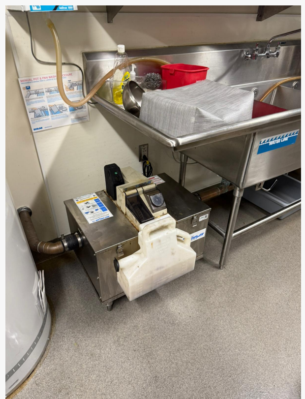
A well-maintained grease interceptor inside a San Bernardino restaurant kitchen helps prevent sewer blockages and supports local FOG compliance standards.
