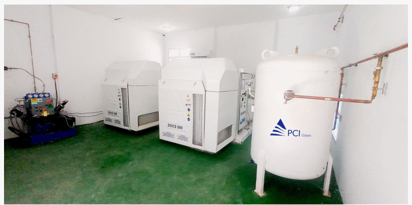
Installation of 2 x DOCS 500 Medical Oxygen Plants at EFSTH The Gambia
