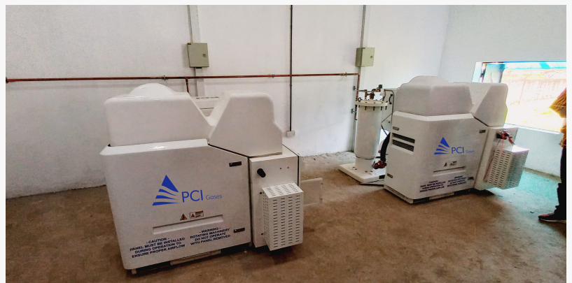
Installation of 2 x DOCS 80 Medical Oxygen Plants at F.J. Grante Hospital Greenville Liberia.
