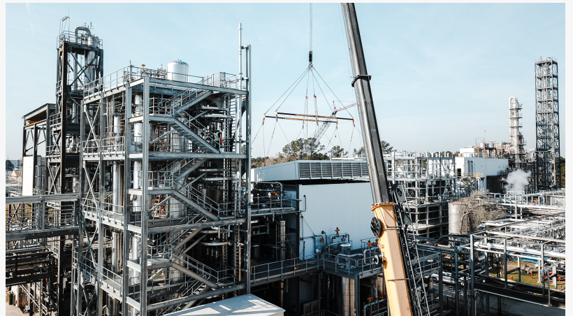
Bushy Park Industrial Complex, Symrise Chemical Process Plant
