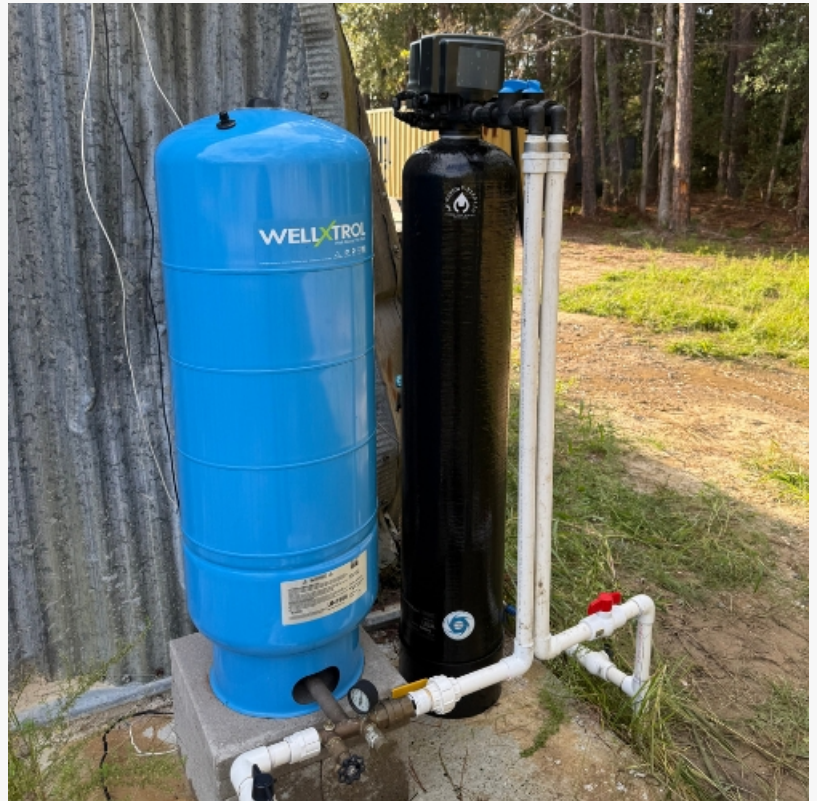
A freshly installed well pressure and filtration system keeping Mississippi homes flowing strong.
