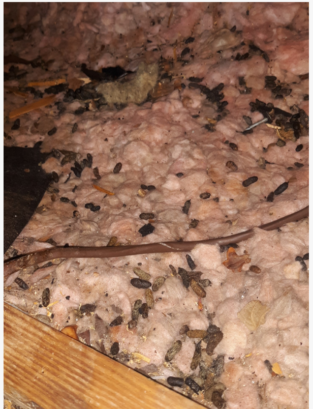
Rodent Entry Point in Vent
