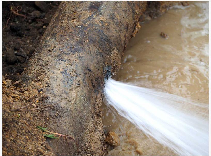
High pressure water main break
