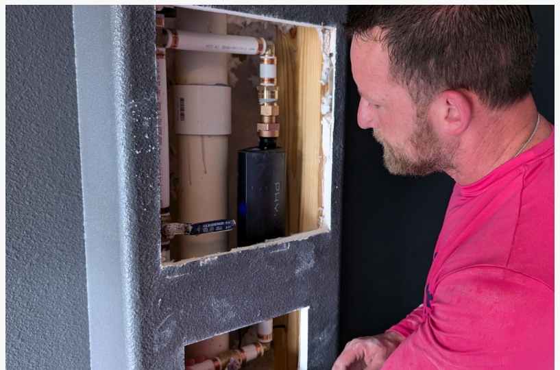
Mother Modern Plumbing installs Phyn Plus Smart Water Assistant in Dallas home.
