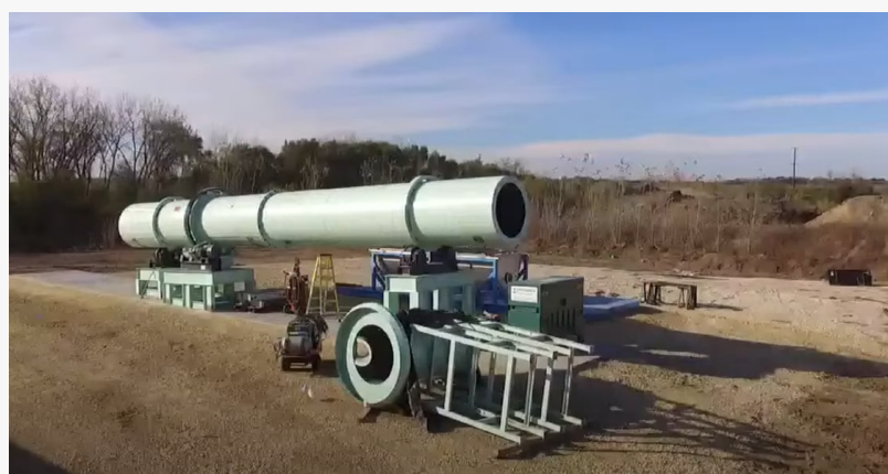
Equipment installed at the Burnsville Biocarbon with Landfill Burial Project
