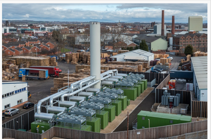
Terra Firma Energy Burtonhead Road 20MW Flexible Generation Plant St. Helen's UK.
