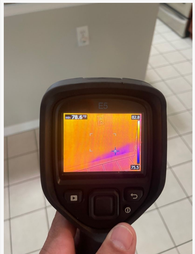
SERVPRO of Fort Pierce NE uses professional thermal imaging equipment to locate hidden moisture behind walls and floors during water damage restoration.
