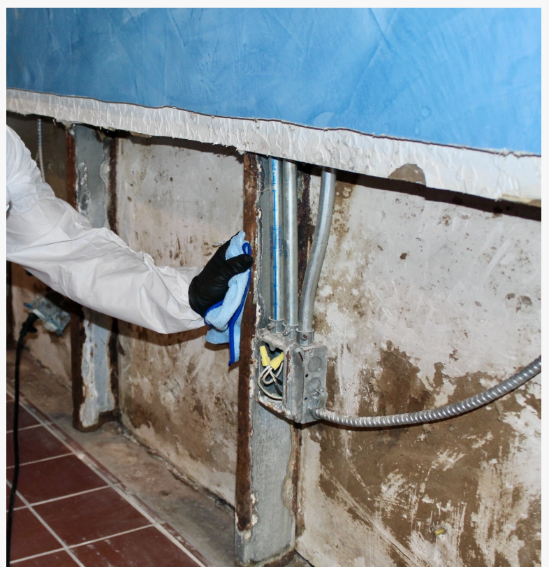
A flood cut in progress as part of the water damage restoration process, allowing affected wall materials to be safely removed and dried.
