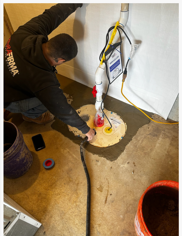
Ensuring active drainage systems, like this TripleSafe™ sump pump, are fully operational is a critical step in protecting homes from shifting soils after heavy rainfall.
