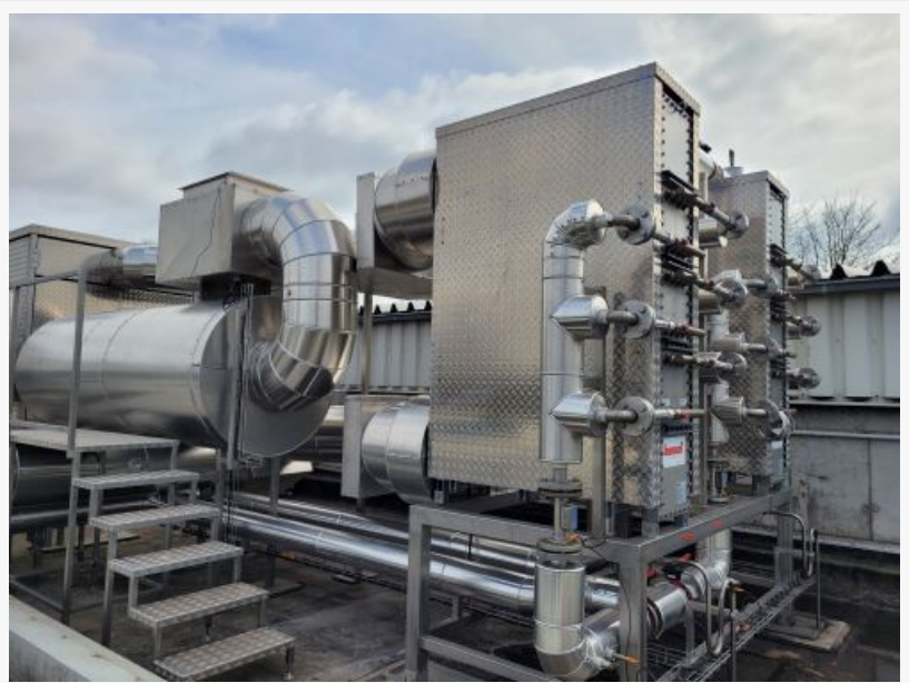
A biogas plant in Northern Germany is shown with the BOMAT heat exchange system
