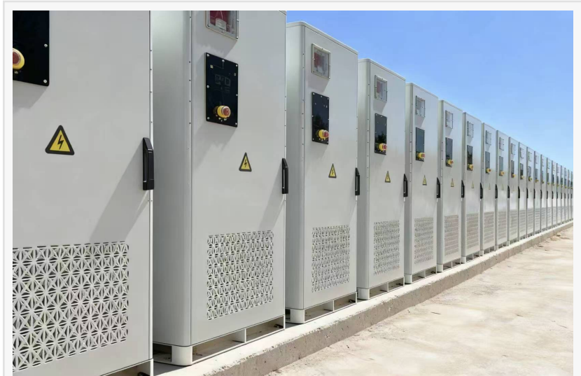
FFD POWER BESS
