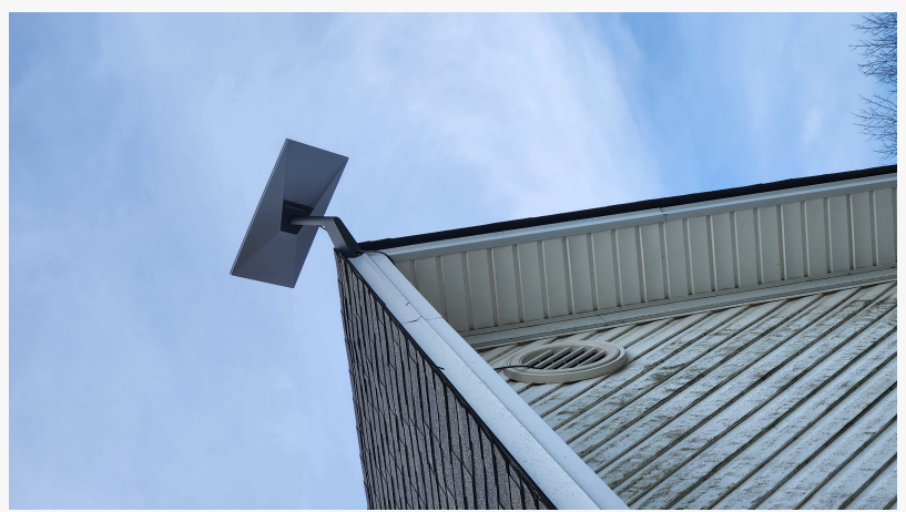
Starlink installation routed through the attic by DishNinjas to ensure clean cable management and a professional finish.
