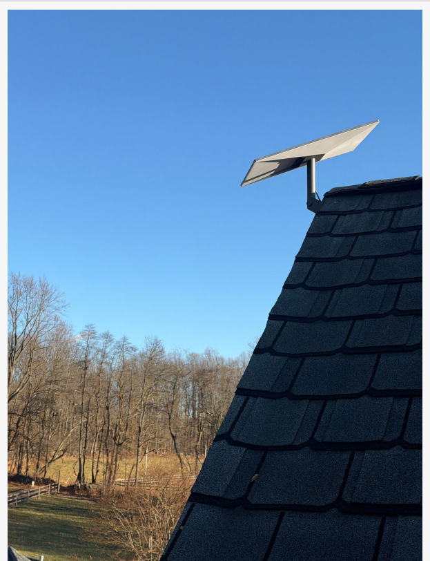
Professional Starlink installation by DishNinjas for residential and commercial customers across the United States.
