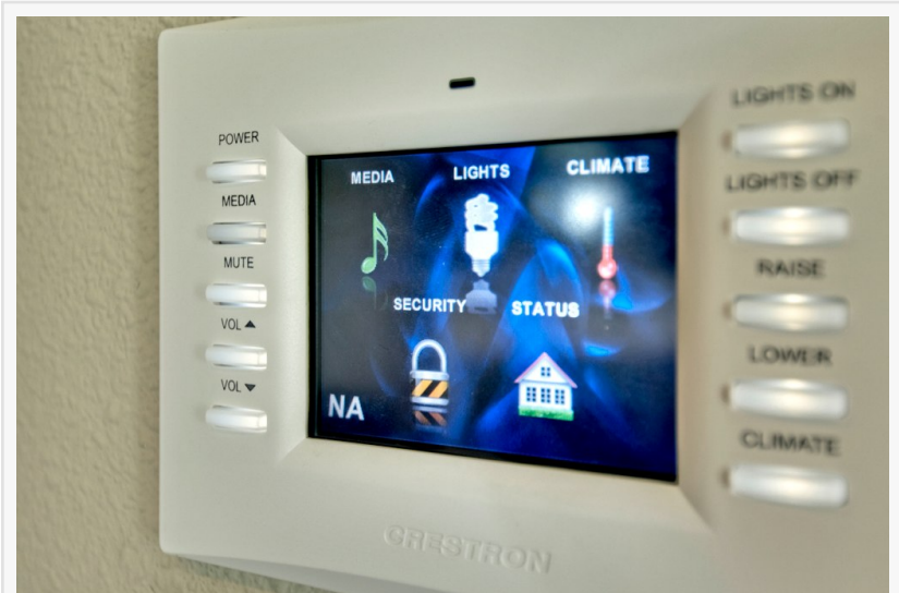
Smart Home Integration Touch Panel Installation
