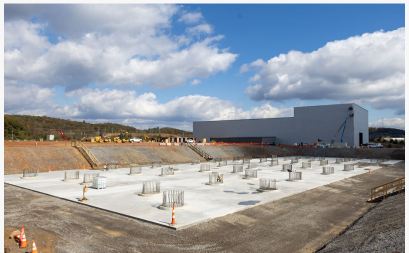
Caption: The Hermes Low-Power Demonstration Reactor is under construction in Oak Ridge, Tenn.
